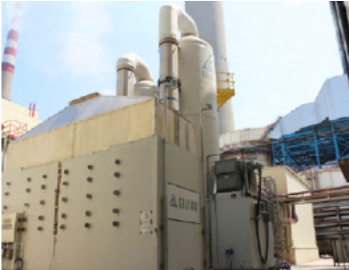
Gradiant’s CGE unit concentrating power plant FGD wastewater
